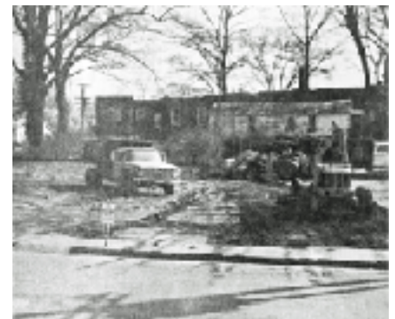
THIRTY YEARS AGO this was the site of one of the finest hotels to be found in this area. A few months ago workmen began tearing down the old Jessica Hotel which was noted far and wide for its fine meals of years gone by. Wednesday workmen began hauling in gravel and construction of a new display lot for Word Motor Company began.
