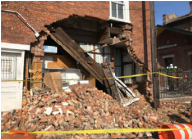
December 2017 just after the train accident
